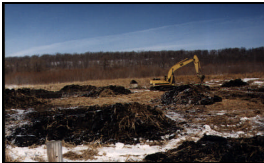
Island Construction Area & Nesting Structure Figure 57 USACE St. Paul District Photo taken by Tim Bertschi
