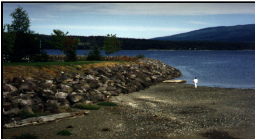
Riprap (Full Bank) Near Sequim, Wash.
