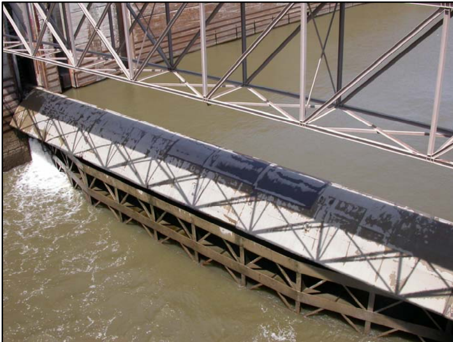
Lock 27: Serious fatigue damage to original main chamber upstream lift gate leaf.
