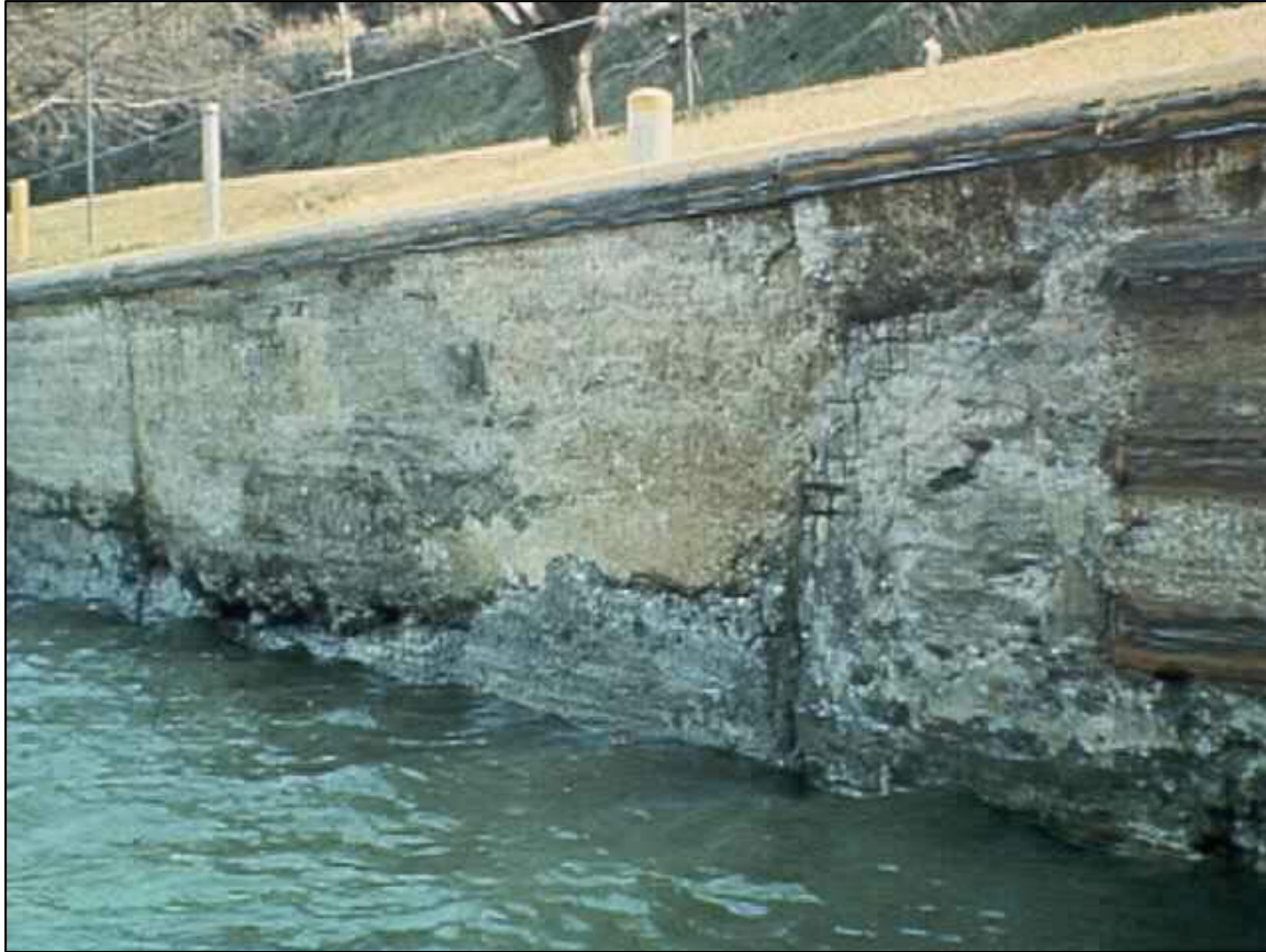
Crumbling Lock Wall on Lower Mon 3, opened in 1907
