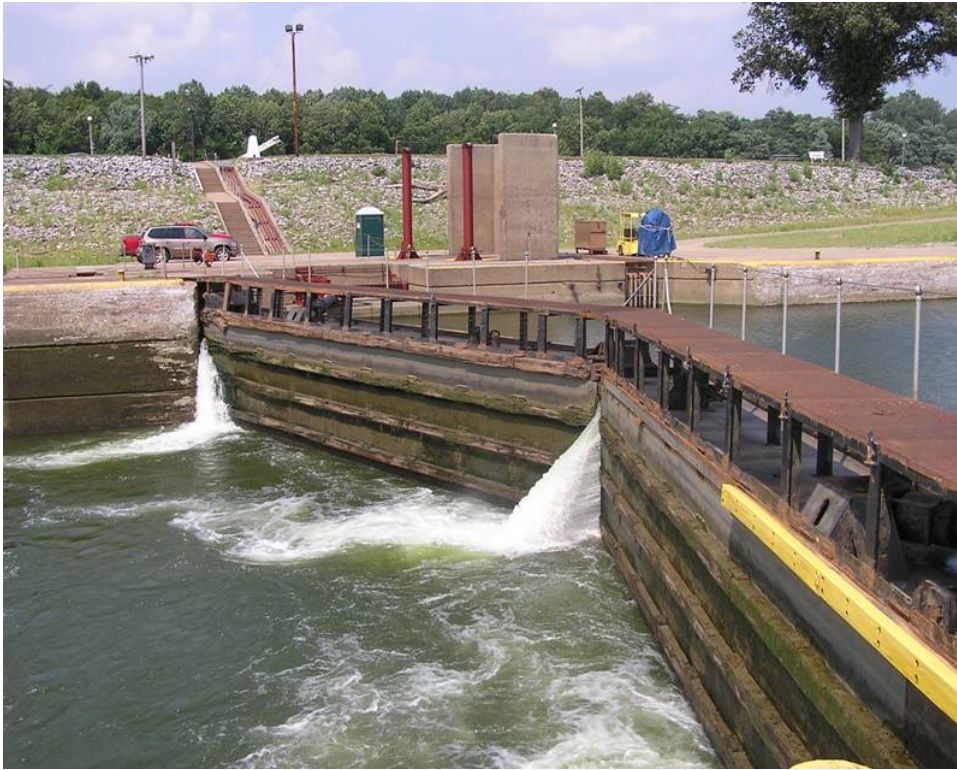
Leaking Miter Gates at Lock and Dam 52 on the Ohio River Olmsted Lock and Dam will replace this facility.
