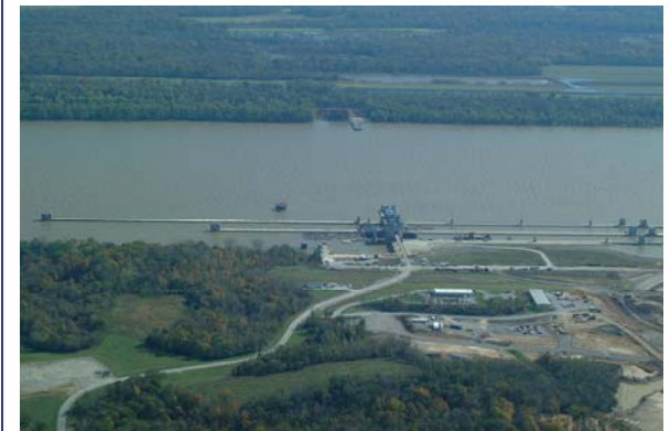
Olmsted Locks and Dam Project, Ohio River New Locks await construction of dam.
