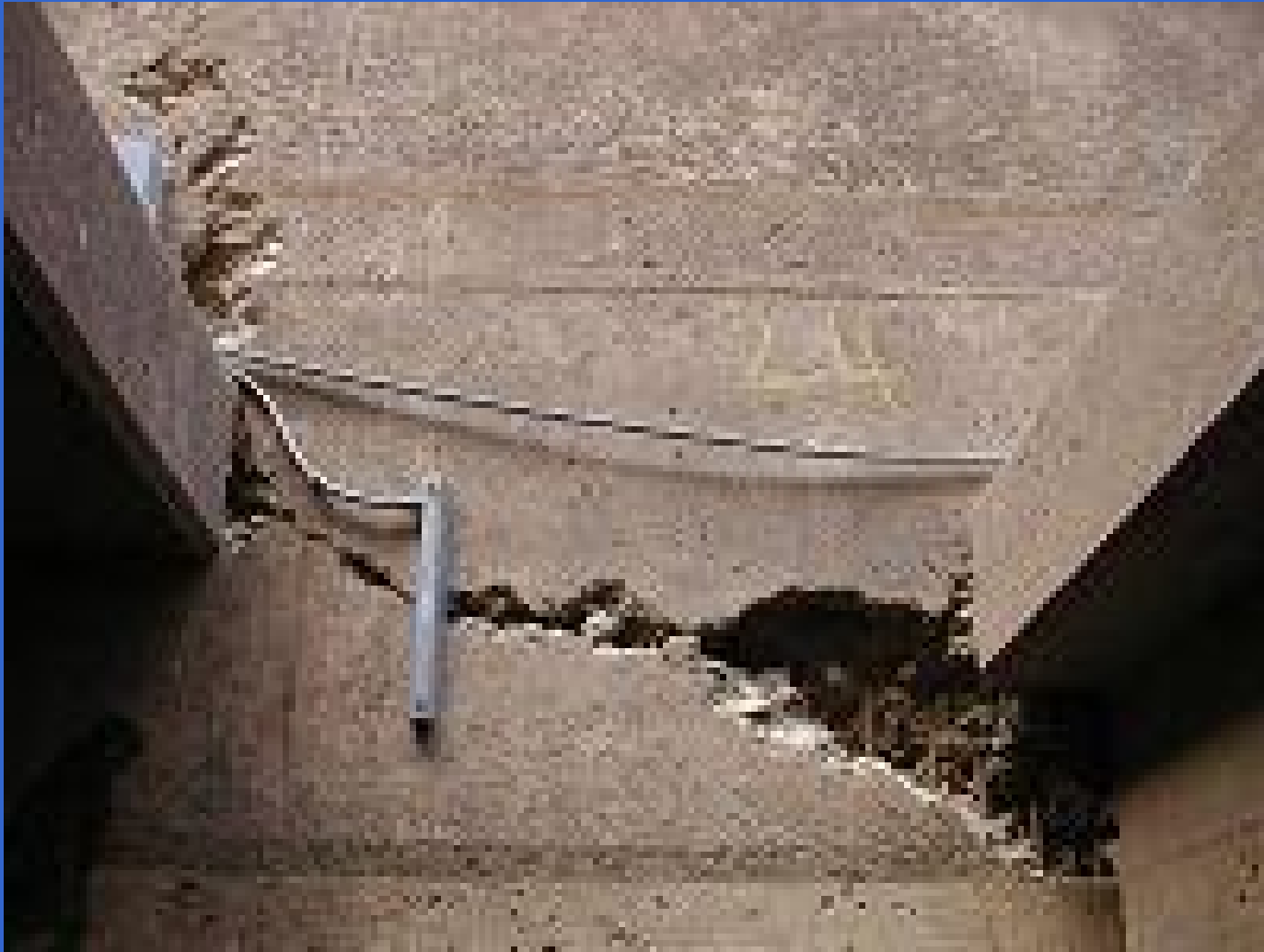
Horizontal Cracking on Monolith bases
